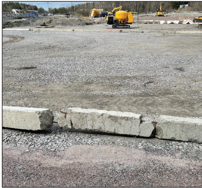
Figure 2. Example of a damaged pile due to encountering of boulders while driving into the soil.
