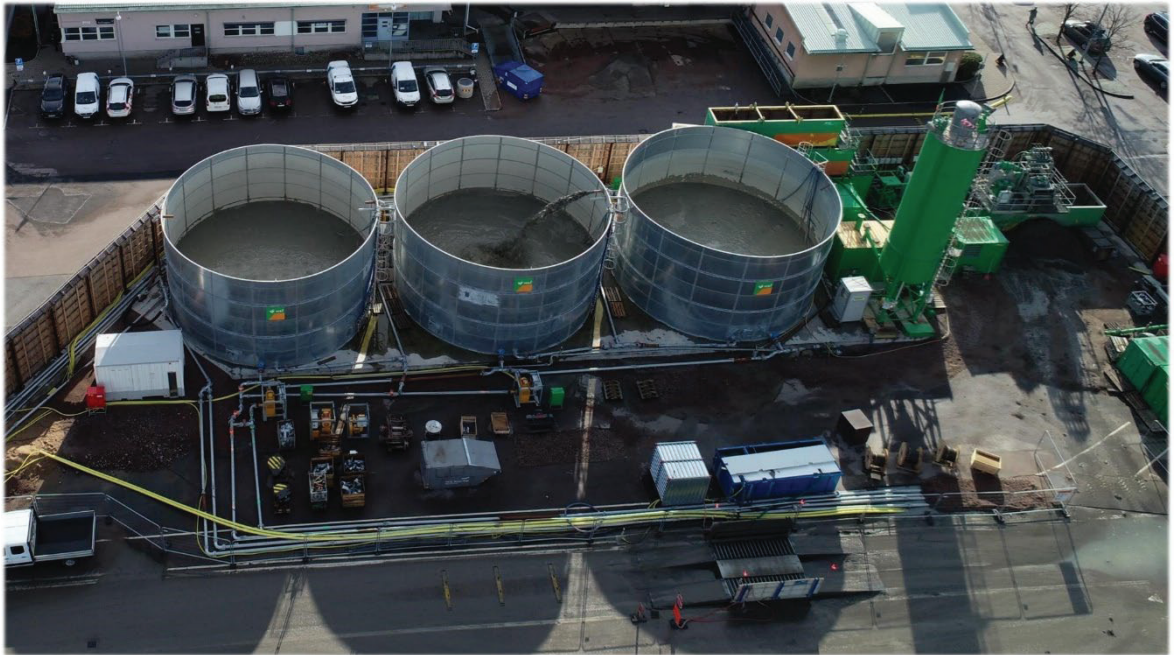
Figure 9. Mixing and reprocessing plant
