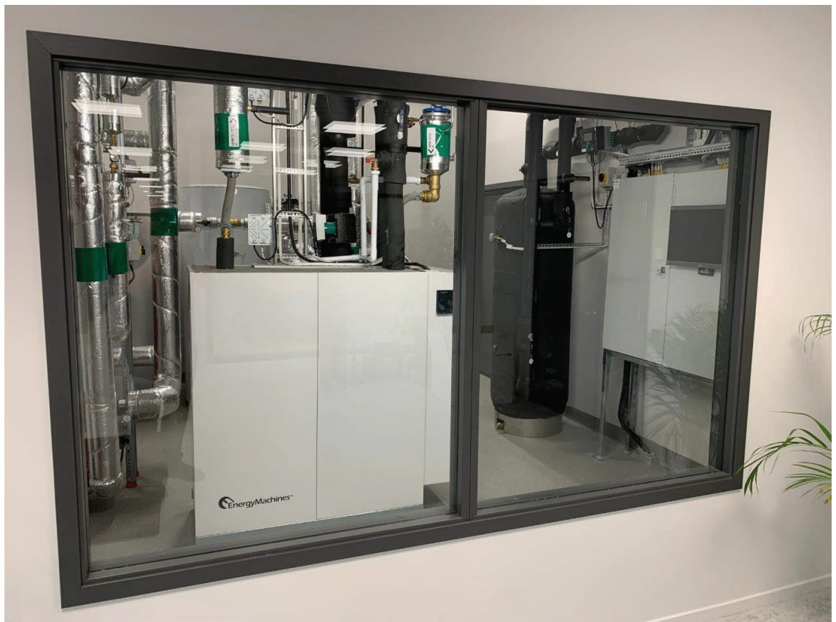
Figure 8 - Final energy central in Centrum Pile HQ. The heat pump is seen in the front. The screen on the right shows live data about the system's performance.
