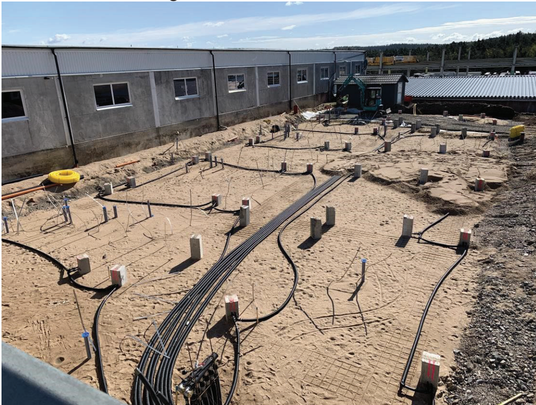
Figure 7 - Connecting precast energy piles in series for Centrum Pile HQ. Property of Centrum Pile AB.
