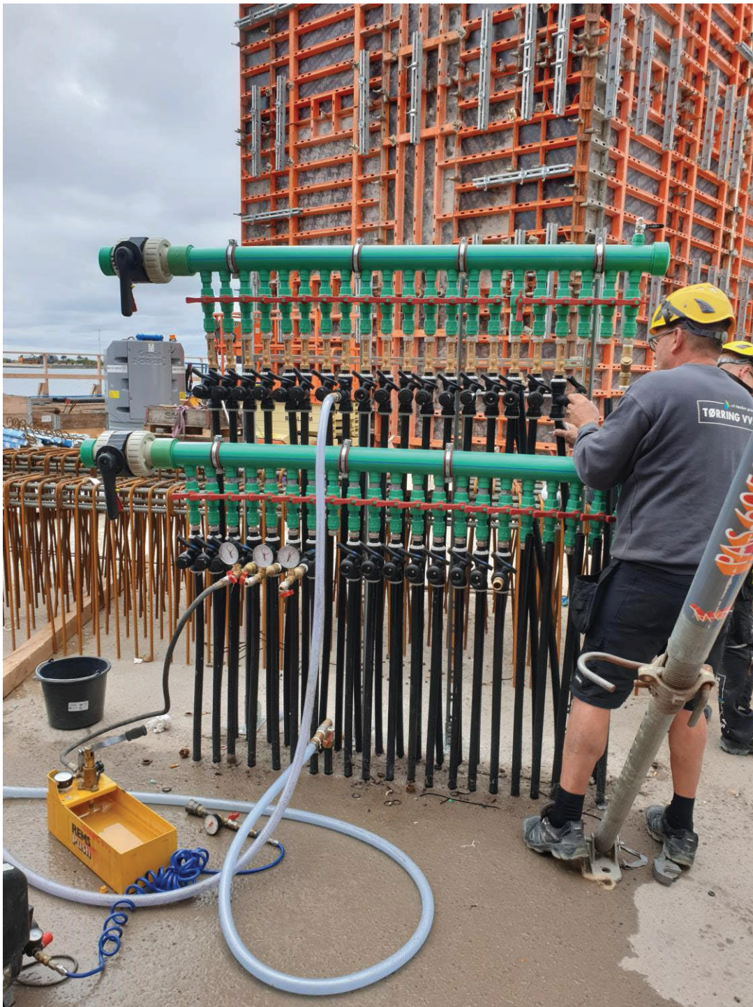
Figure the heatpump. Property of Centrum Pæle A/S.5 - Central manifold for energy pile in- and outlets, which will ultimately connect with
