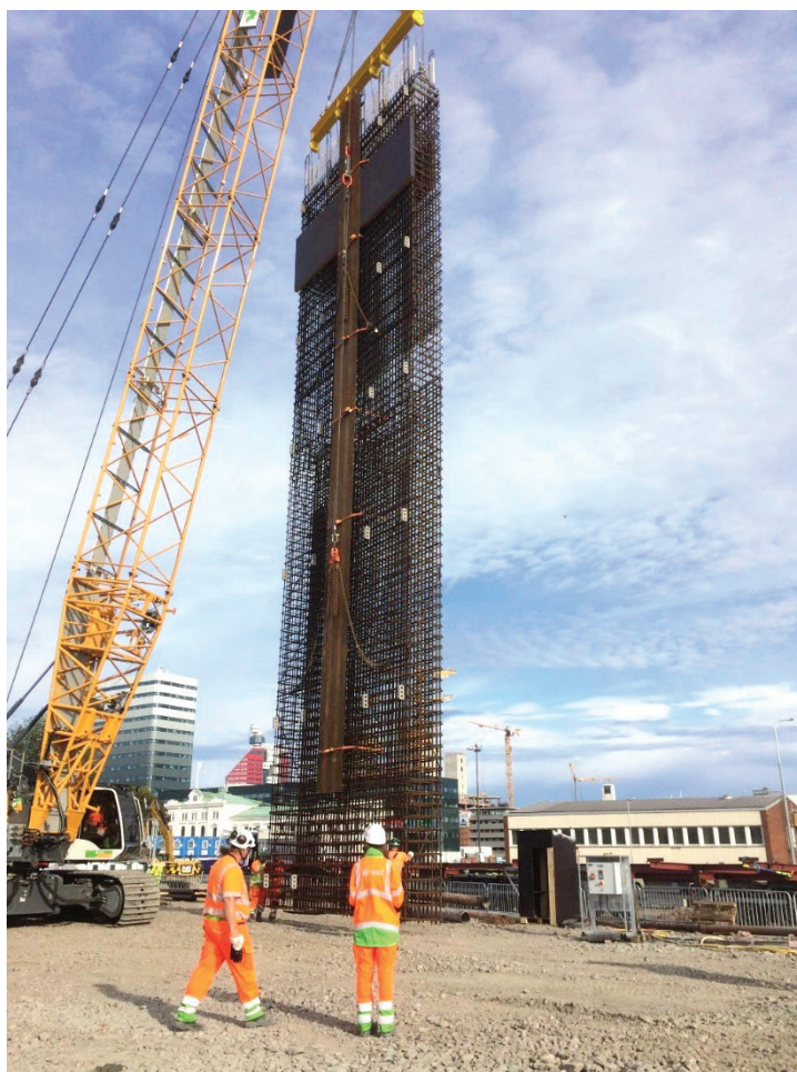
Figure 10. 40 tonnes reinforcement cage connected by a special lifting device to a crawler crane. Central steel joints enables the cleaning of the cross wall connection.
