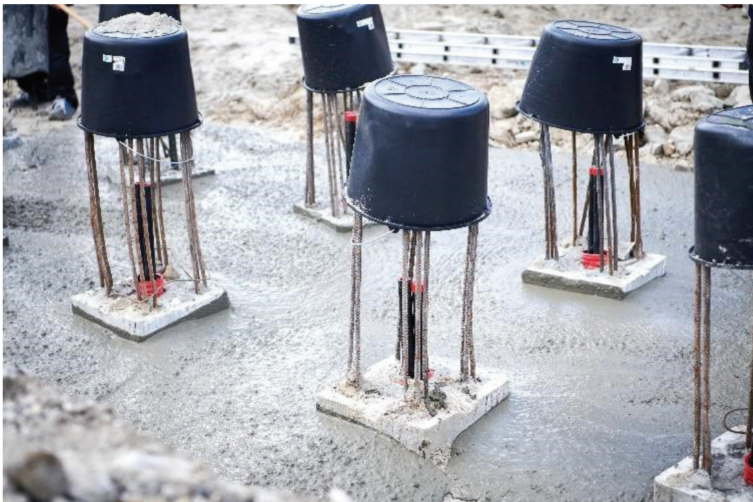
Figure 3 - Installed precast energy piles, ready for series connection. Property of Centrum Pæle A/S.
